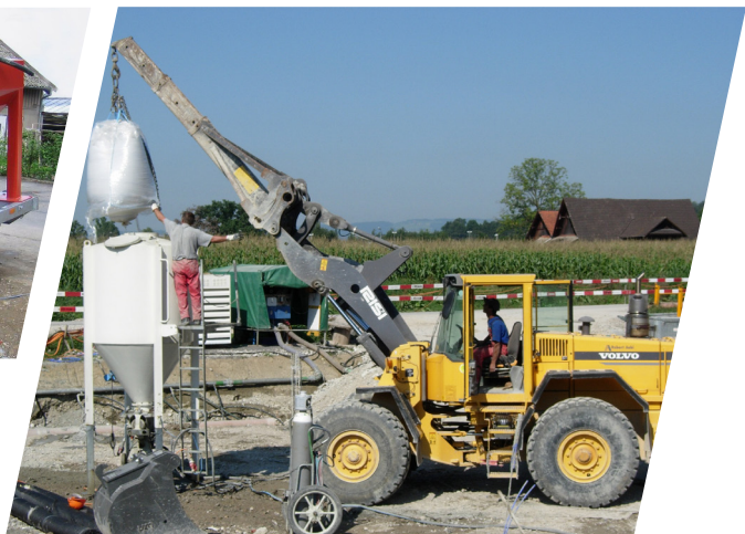
Filling the silo using the BIG BAG
