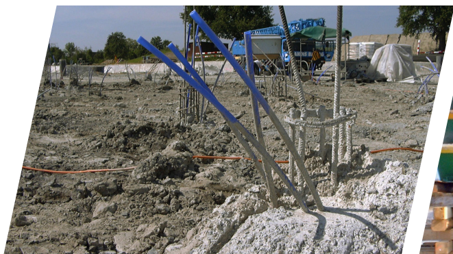
Upper concrete pile with four pieces K Injection lines deployed in two different depths
